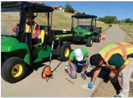
Facilities staff Paula Horsley and Dave Watson installing 1/4-mile trail markers with TEP team member Brenda Bowcut
