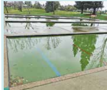
Ponding on the courts; no boogie boarding allowed
