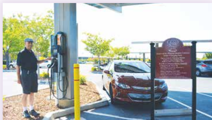
Ken Silverman prepares to charge his vehicle using the Electrical Vehicle Charging Station
