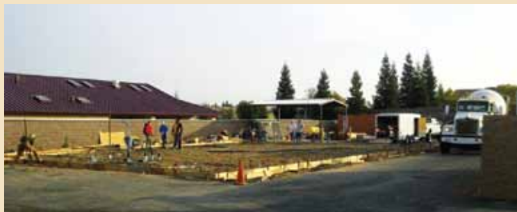
Foundation for Maintenance Building installed in November, ready for erection of pre-fab metal structure
